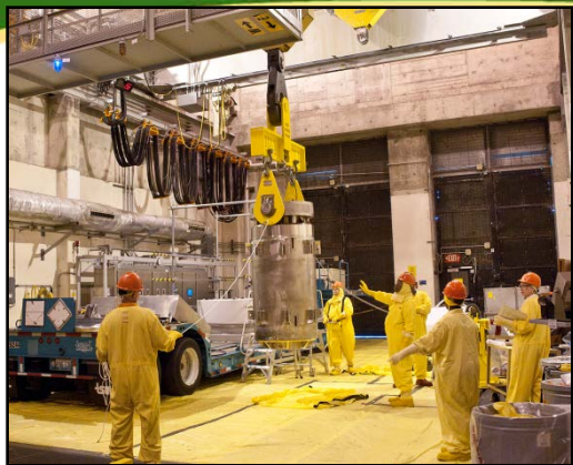
Receive Cask/ Removed Impact Limiters
