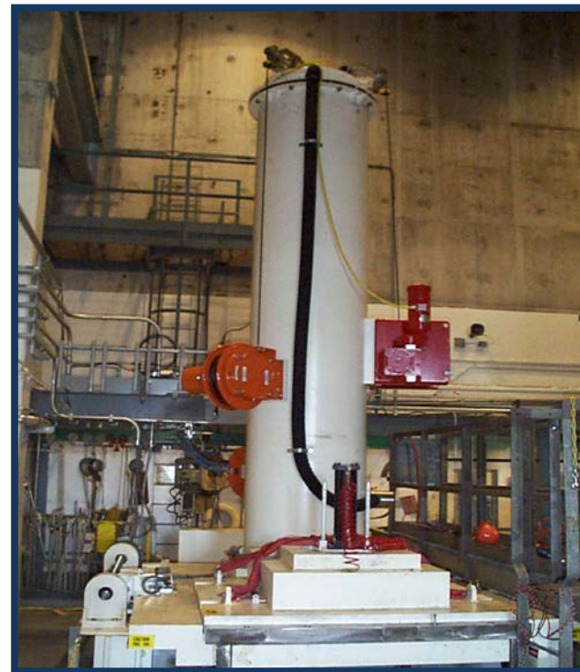
Shielded Transfer System (STS)
