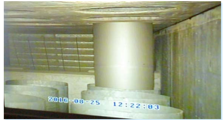
Inside View of Vault A - Double Stack
