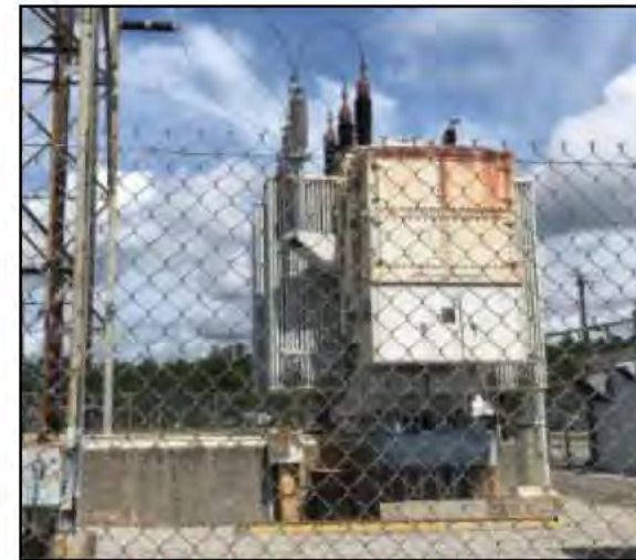
K-Area 151-1K Substation Transformer Today
