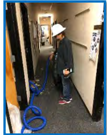
Interior Damage in 766-H Training Building
