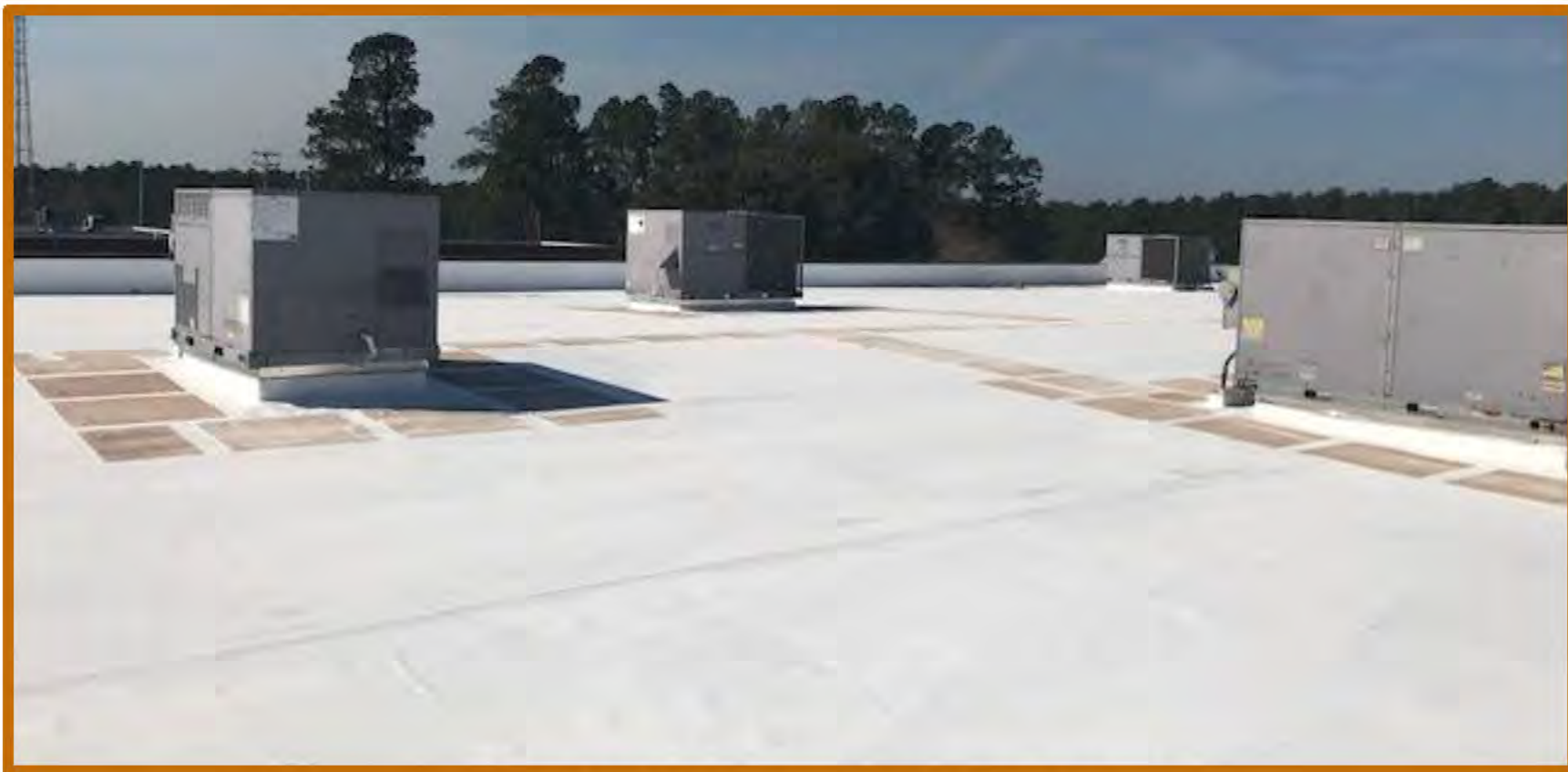
703-47A New Eco-White Cool Roof
