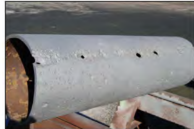
Galvanic Corrosion in 70 Year old Service Water Pipe
