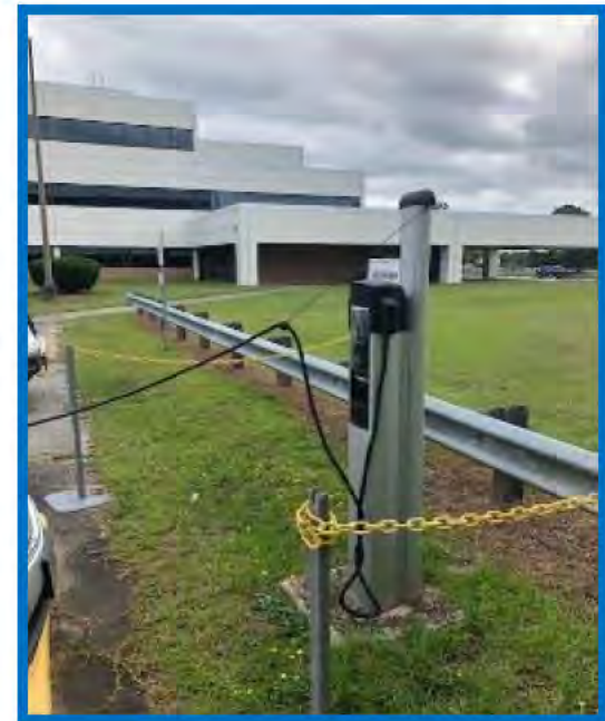
B Area EV Charging Station
