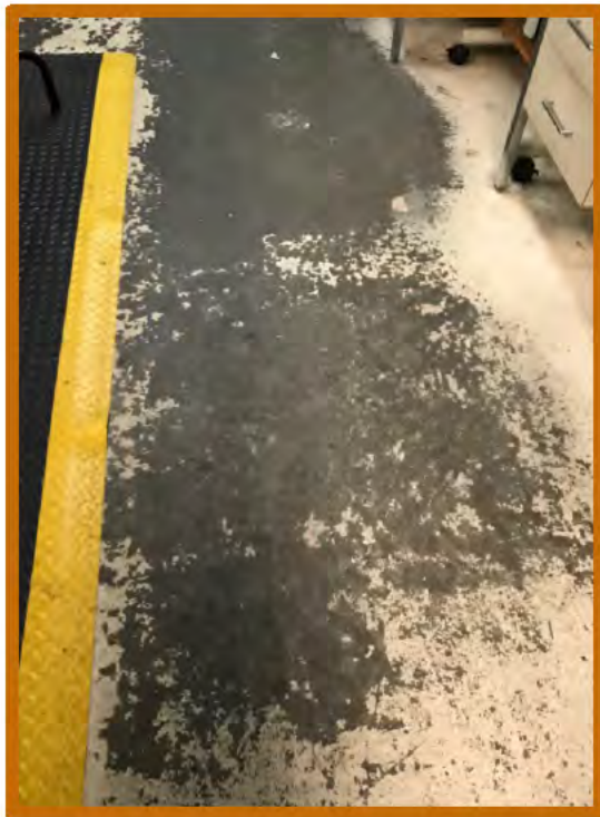
703-5B Chipped floor coating
