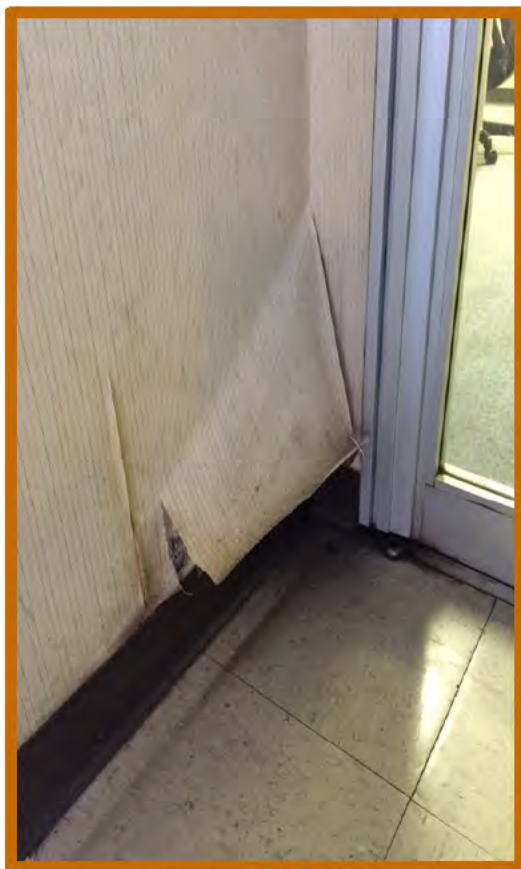
703-42A Water damaged wall coverings
