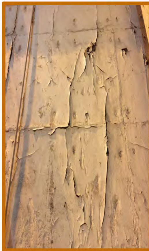
717-F Degraded shop wall insulation
