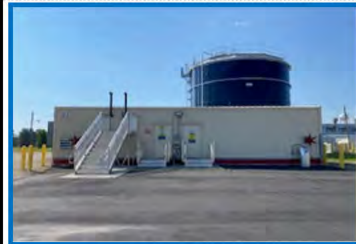
New A-Area Firewater Water Pump House and Tank Completed 2020
