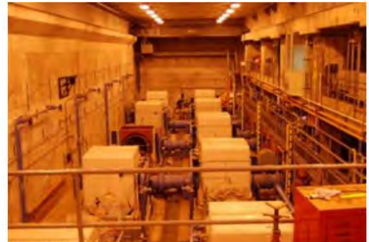
River Water Pump House 681-3G
